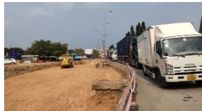
Road in Buffer zone of Bavet Border is widened by MPWT, Cambodia (Vietnam Border)
