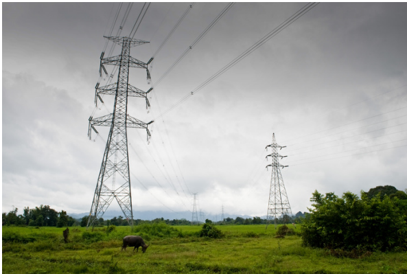
Power transmission lines from the Nam Theun 2 Hydropower facility.
