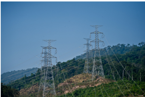
The taller power lines delivers 500kV of electricity to Thailand, while the smaller mast delivers 115kV of electricity for domestic use.
